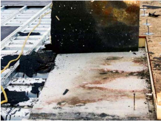
Figure 3. Mold growth in roof insulation caused by air leakage.
